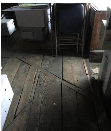
Uninsulated floor in attic
