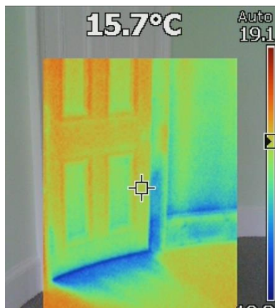
A cold draught showing under internal (MCB board) cupboard in stairwell
