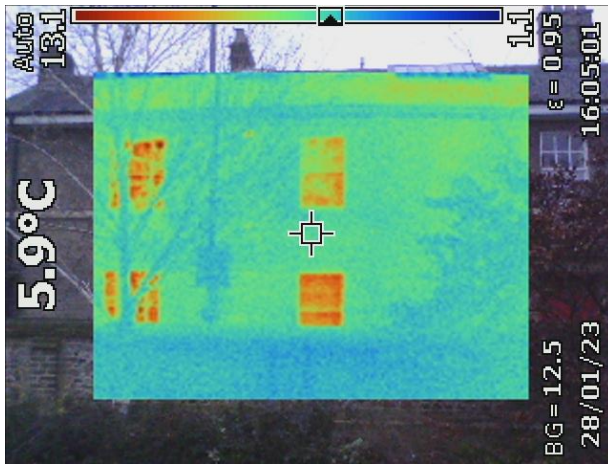
Again, in this image of the Bateman Street side of the building, you can see heat leaking mostly through windows but also through walls and roof
