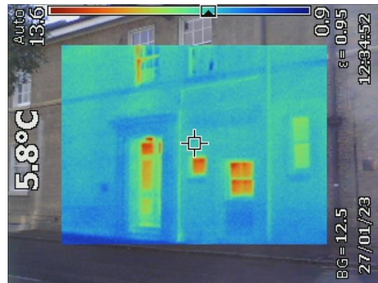
Main entrance from exterior, with heat loss seen through single glazing and wood panelling of door and windows
