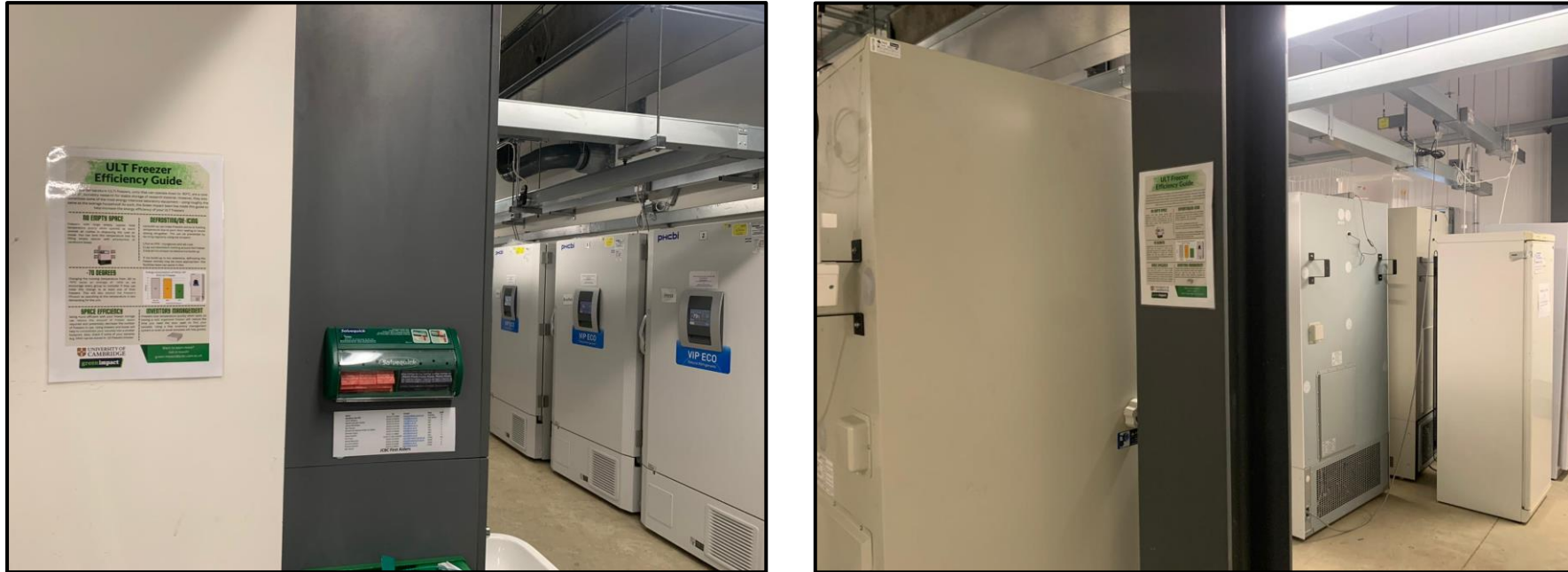
Evidence of our freezer efficiency guide on the walls in the freezer room
